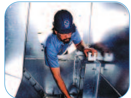
Electric water level control
